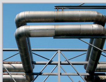
Pipelines subject to pressure
